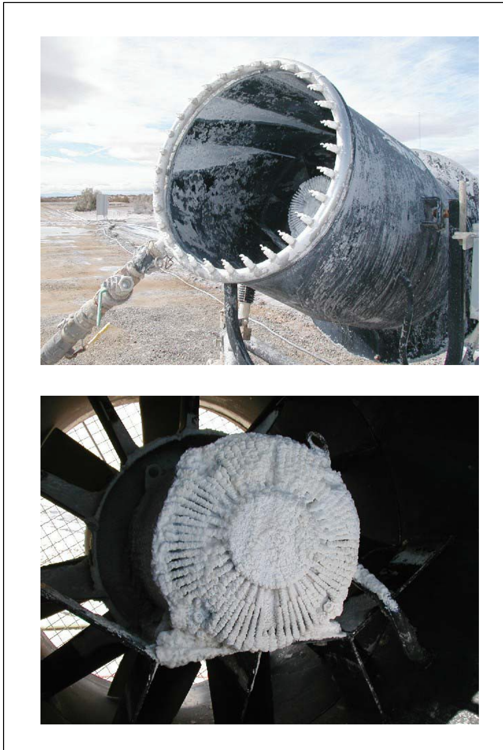
Figure 5.8—Salt deposits on evaporators from mist ingestion.
